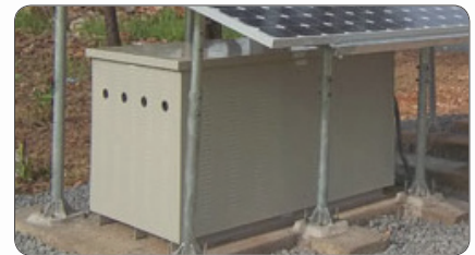
Kotak Battery Bank Outdoor
